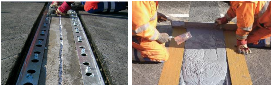
Figure 12: Fixing angles to polymer concrete base (left) and precise levelling to road surface (right)
