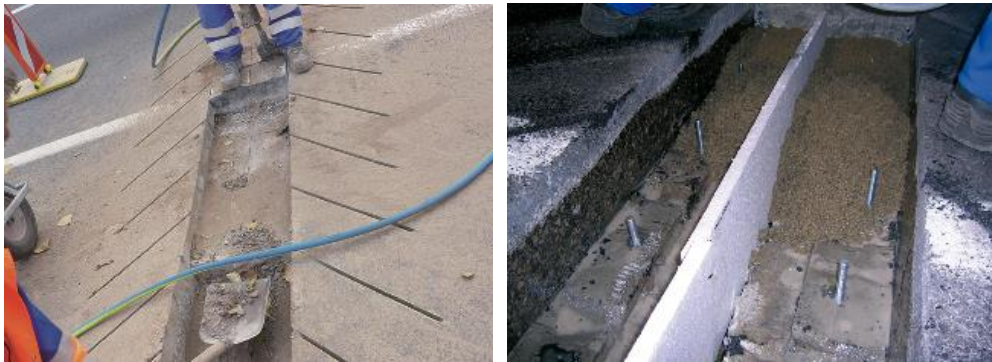
Figure 11: Removal of old joint/surfacing as needed (left) and forming of polymer concrete base (right)
