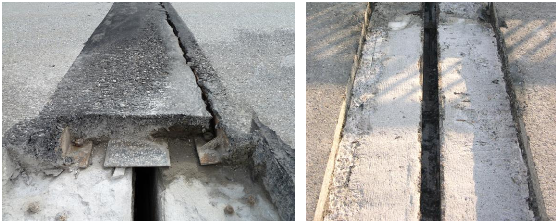
Figure 2: If installation of a new expansion joint as a replacement for an old existing joint, such as that shown on the left, requires the removal of existing joint/structure only within the depth of the structure's asphalt surfacing, as shown on the right, the work can be substantially accelerated
